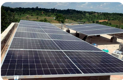
Flat-roof commercial solar array
