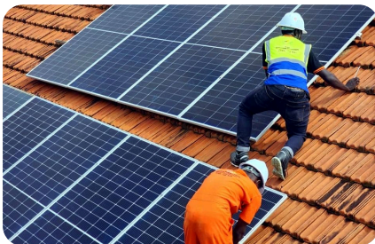
Rooftop solar array on a tiled roof
