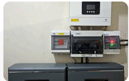
Hybrid inverter and lithium battery installation
